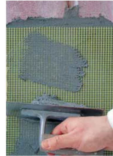
(5) Application of rialto fibralarge and subsequent application of second coat of leveling product
