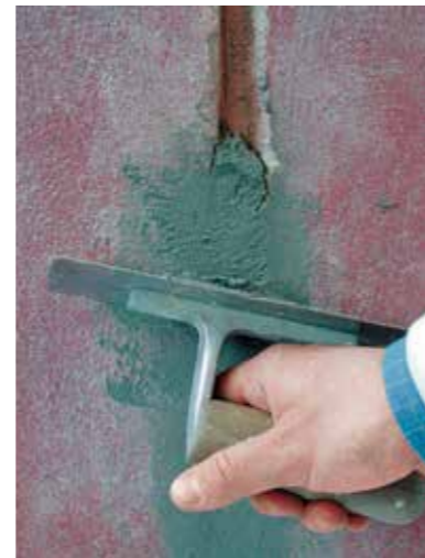
(3) Sealing the crack with cement mixture based on rialto intonal or matonal
