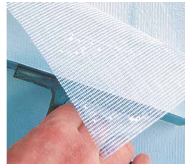
(1) A dry and clean cracked surface
