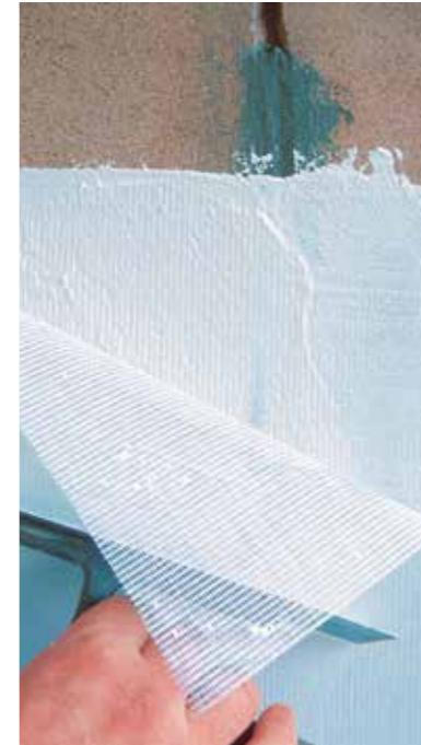
(5) Application of rialto fibralarge and leveling treatment with second coat of rialto raselast
